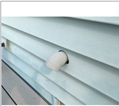
Example of utility penetration needing caulk
