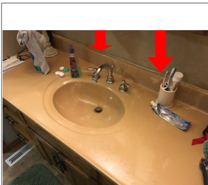
Loose countertop/bad caulk joint
