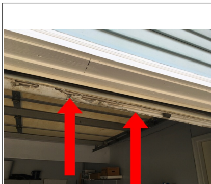
Weatherstripping is damaged on garage door
