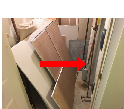
TPR valve not extended far enough on State water heater
