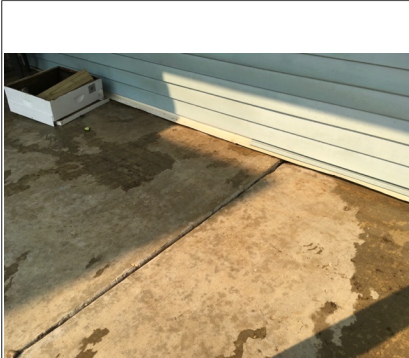
Uneven slab on porch
