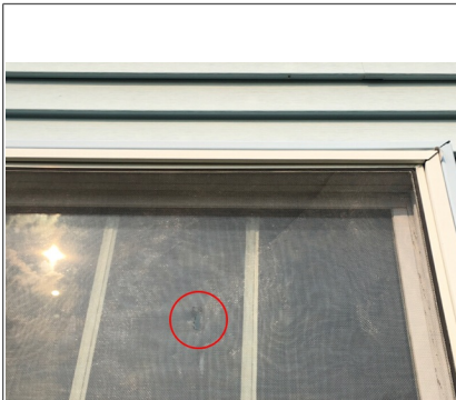
Example of a torn and bent screen (garage window)
