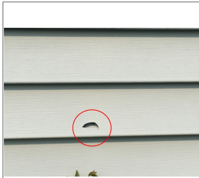
Example of cracked hole in siding
