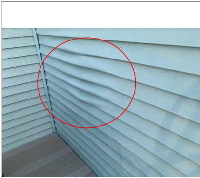
Siding warped from excessive heat by grill sitting on deck.
