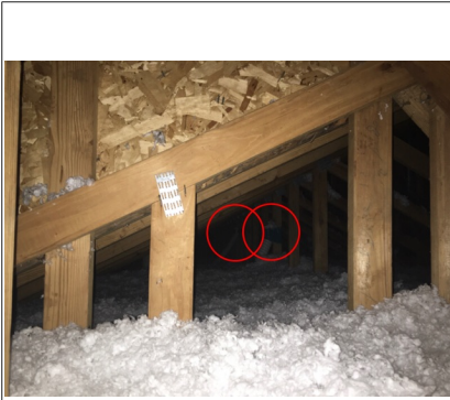
Two bath fans not vented to the exterior
